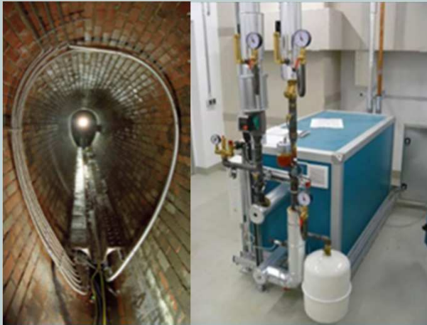
Waste-Water Heatpump (2 x 22 kW)
